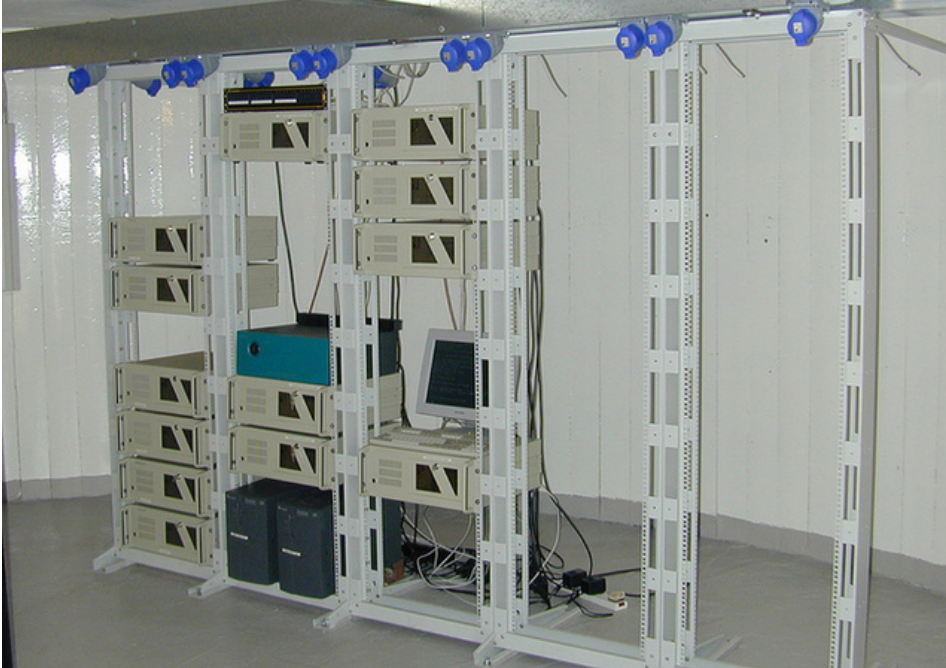
The Sealand data center (later moved off the fort to London)
